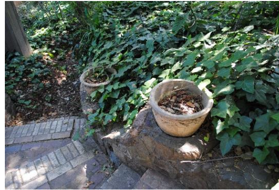
Figure 166. Staircase paved with Carnegie bricks, flanked by masonry retaining walls with ceramic pots.
