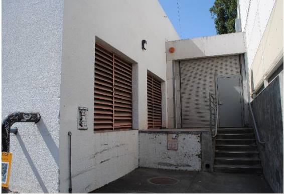
Figure 143. Metal roll-up door accessed via concrete steps on the north side of the hyphen between Barclay Simpson Sculpture Studio (right) and the Shaklee Building (left).
