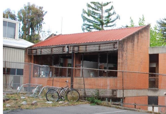
Figure 107. Ceramic Arts Center, portion of east façade with shed roof, looking southeast.
