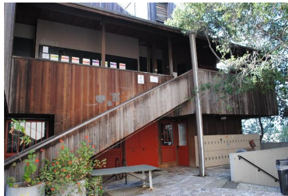
Figure 67. Martinez Hall, primary façade detail, south portion of the first and second stories, facing southeast.
