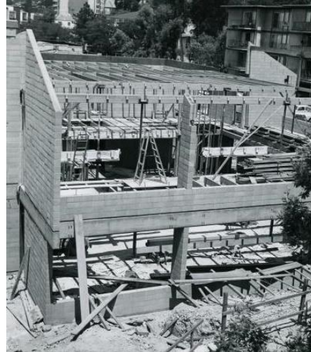
Figure 112. Site clearing and construction of the Noni Eccles Treadwell Ceramic Arts Center, 1973. Source: CCA Libraries Special Collections.
