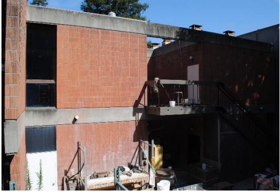
Figure 108. Ceramic Arts Center, portion of east façade with concrete balcony and stair, looking northwest.
