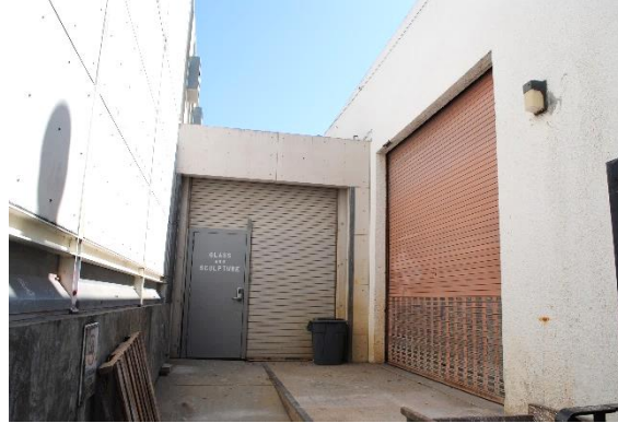
Figure 123. Large metal roll-up door at the south end of the west façade of Shaklee Building (right), looking south. A hyphen addition attaches to Barclay Simpson Sculpture Studio (left).
