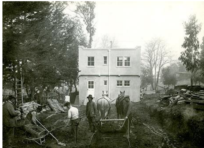
Figure 42. Students and other laborers clearing land for the construction of the craft building (B Building), south of the completed woodworking studio (Facilities Building), 1925. Frederick Meyer is visible at the lower left of the photograph. Source: CCA Libraries Special Collections.
