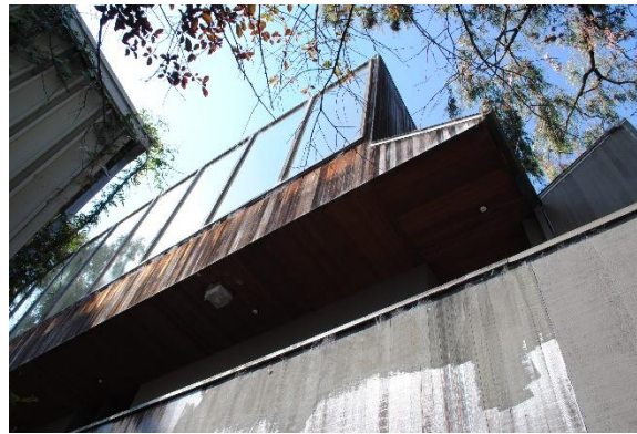
Figure 77. Clerestory windows of the sawtooth roof at the north façade, looking southeast.
