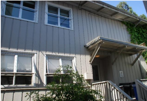
Figure 54. Irwin Student Center, north façade, partial view with secondary entrance, looking southwest.
