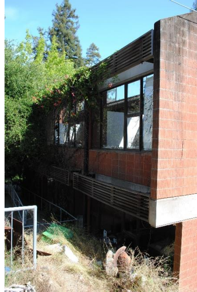
Figure 105. Projecting second story of the south façade, including belt course, wood trellis, and shed roof form, looking northwest.
